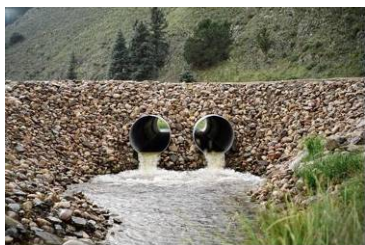
Culverts recently re-installed on the Carson NF with gradient, length, and an apron to provide a barrier to upstream fish passage in Comanche Creek.
